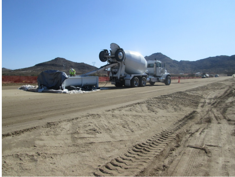
Photo 2: A concrete washout is maintained onsite for cement truck operators to washout equipment in accordance with MM-HYD-1 and the Stormwater Pollution Prevention Plan (SWPPP).
