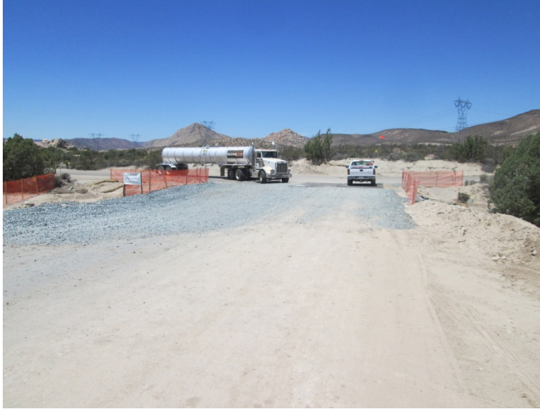
Photo 5: Trac-out measures consisting of a rock apron and rattle plate are being maintained at the construction entrance to the ECO substation along Old Highway 80 in accordance with MM-BIO-4A and the Dust Control Plan.
