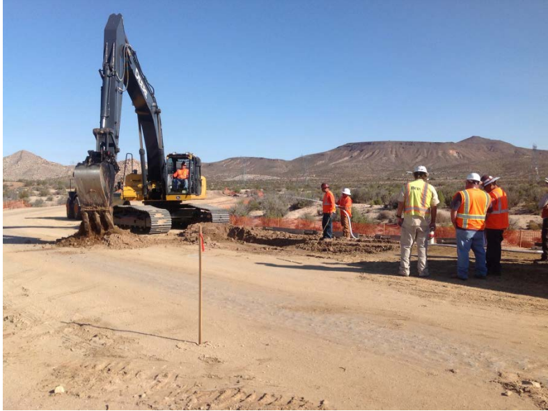
Photo 1: Paleontological, Biological and Archeological monitors were onsite overseeing construction activities in accordance with MM-PALEO-1C, MM-BIO-1C and MM-CUL-1D.
